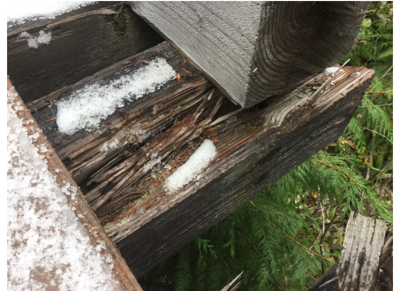
Damage to downstream cross tie
