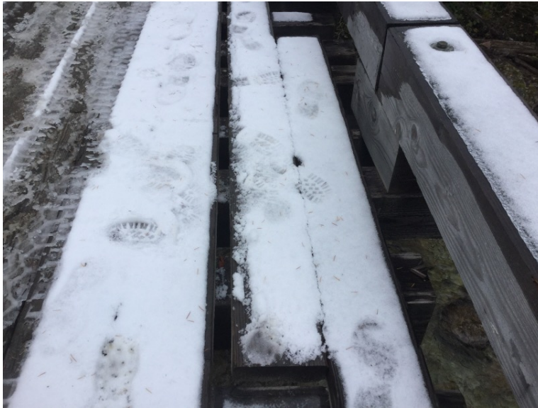
Outside strip of planks on downstream not tight to each other or fastened to cross ties
