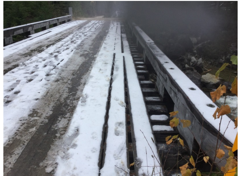
Upstream planks not tight to each other and not fastened to the cross ties
